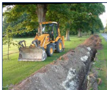
Roots severed and compaction
