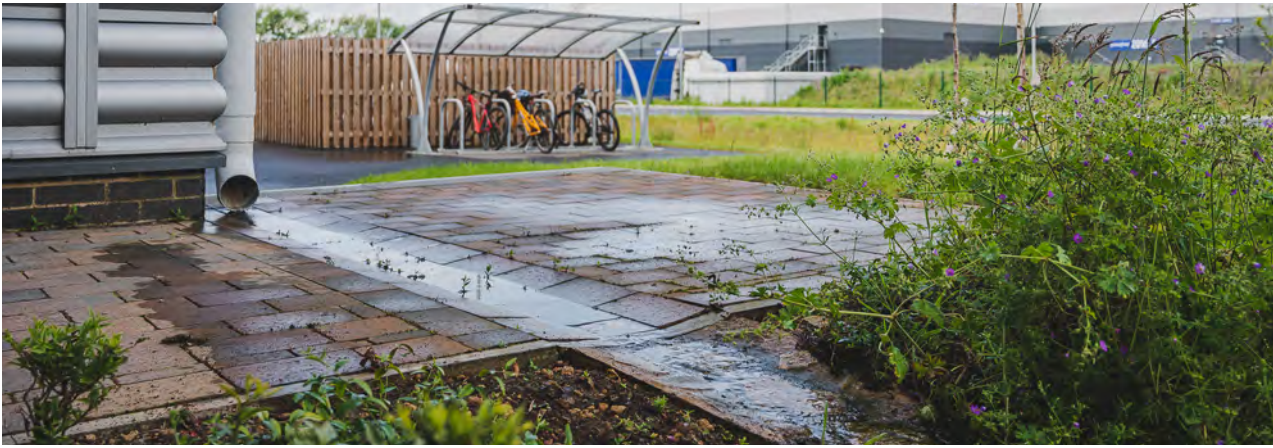
A 'shoe' fitted to a rainwater pipe at the Robert Welch Warehouse, discharges into a paved channel leading to a rain garden.
