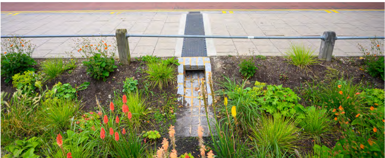
Inlet from road into a raingarden
